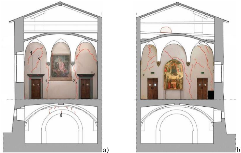
Figure 5: Cracking pattern of the wall containing the fresco (courtesy of Prof. C. Blasi): a) front view; b) rear view.
