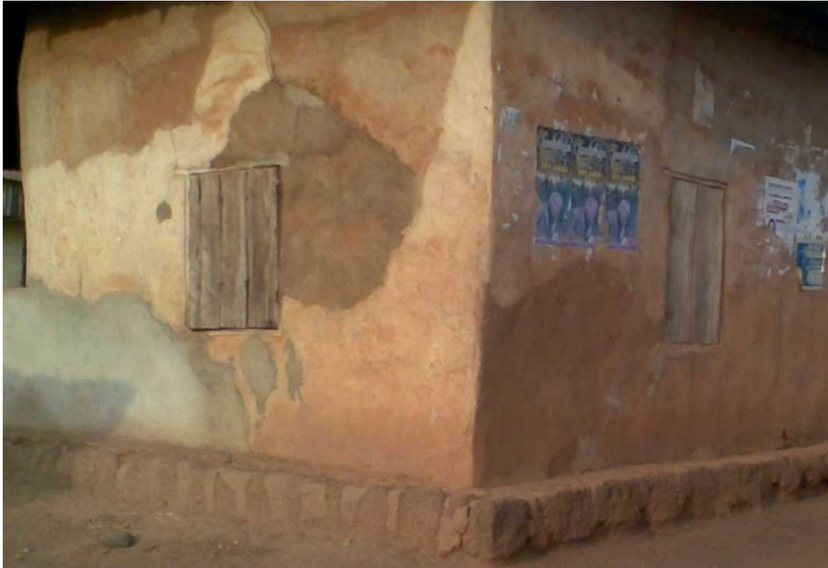
Figure 5: House with Timber Boards over Openings
