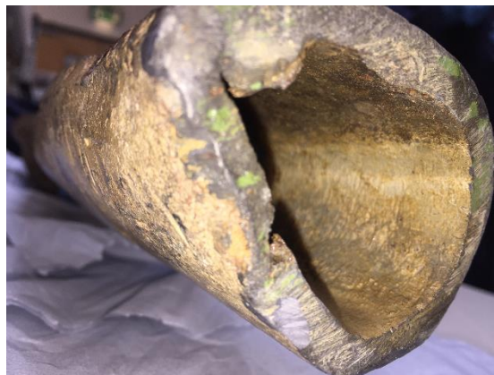
Figure 4: Distinctive sinter line observable in pipe. This indicates a substantial pattern of partially-full flow
