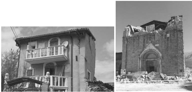
Fig. 2. Examples of out-of-plane collapse mechanisms of masonry buildings.
